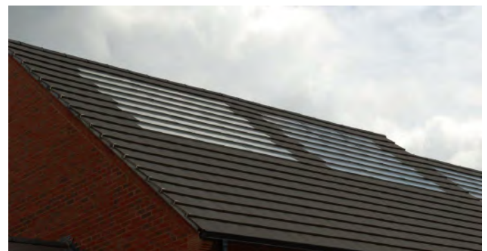
▲ Solar panels are integrated into the roof in Upton. Benefits include, aesthetics, maintenance, safety, and pest control.
